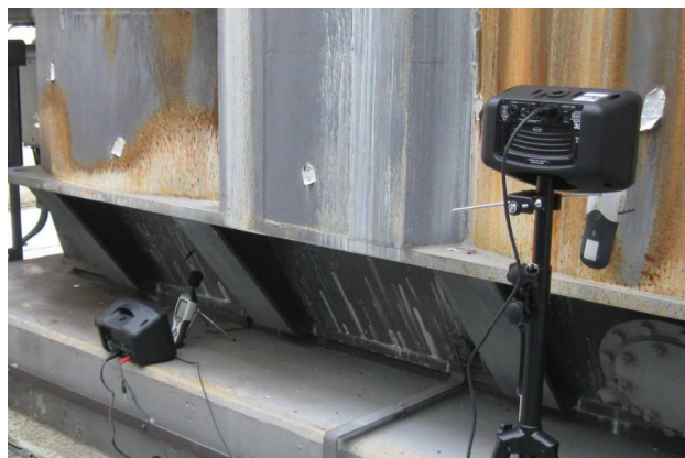
4.1. Speakers at short distance from transformer
