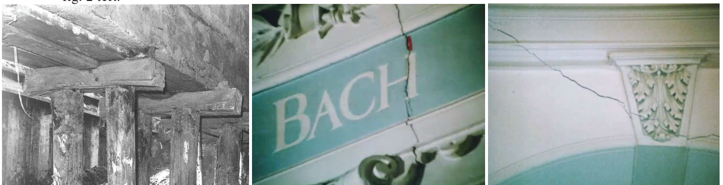
Figure 2. The wooden piles with capping under the building and the cracks in the walls
