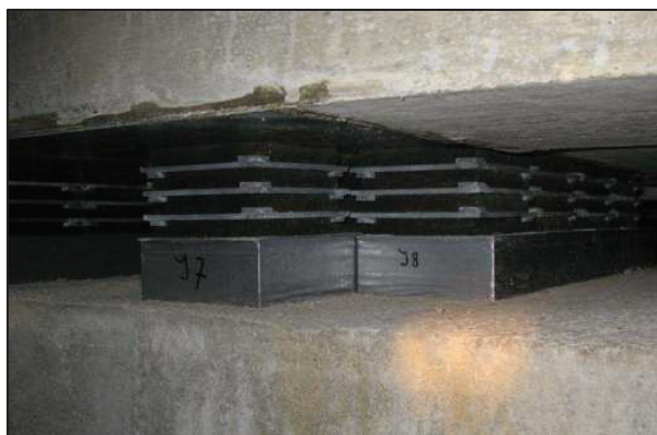
Figure 14. Elastic bearings in position under dwellings on the pop centre during the construction phase.
