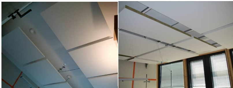
Photograph 3 – Ceiling panels covering 50% (left) and appr. 70% (right).
